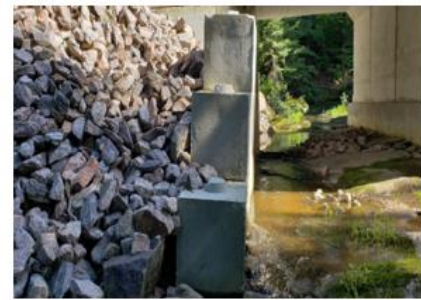
Photo 4: SW retaining wall is leaning towards stream
