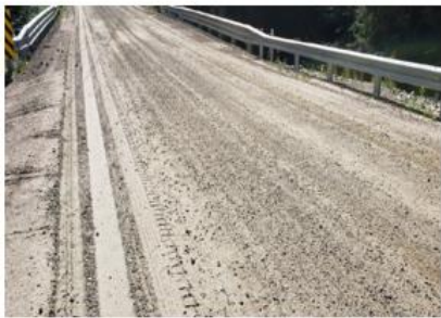
Photo 5: Tire rutting noted on east approach wearing surface
