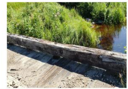
Photo 4: Splits, checks and rot on NW timber curb
