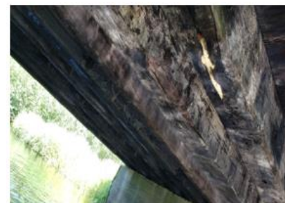
Photo 5: Weathering on timber girders
