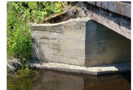
Photo 6: Moderate scaling noted on NW wingwall
